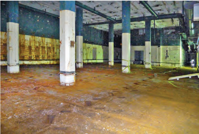
A contemporary photo of the same room. The previous photo was taken from against the rear right-hand wall. All equipment including the raised floor and cable mezzanine has been removed making for a very tall area
